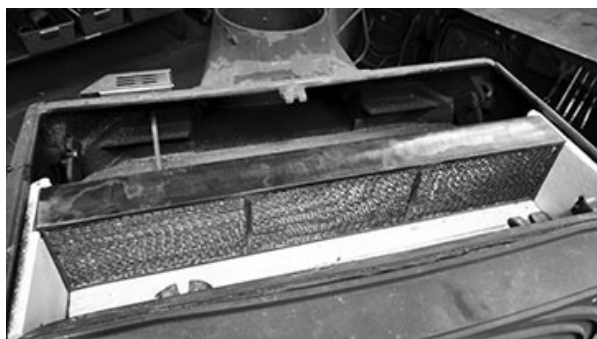
Fig. 23. Lift combustor from the chamber.
