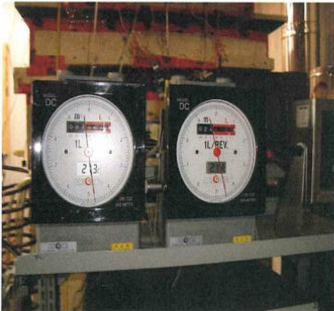
Picture 11: Dry gas meter
